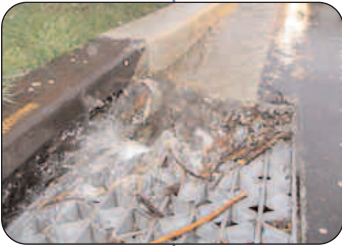
A stormwater drain. (CHESAPEAKE BAY PROGRAM PHOTO)
